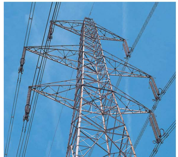
... where electrical energy is distributed
